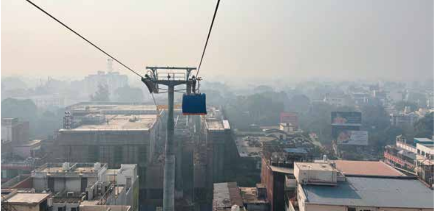
The construction of India's first urban cable car is advancing, with the first test rides having taken place. © BARTHOLET
