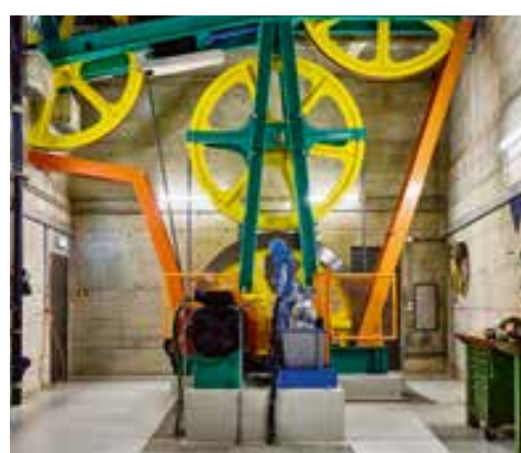
The cable car's technology was extensively upgraded.
